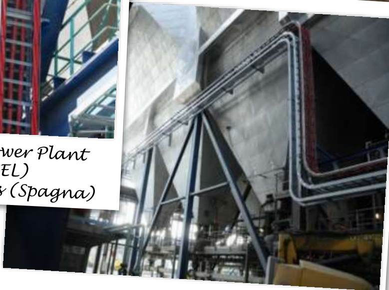
Litoral Power Plant (ENEL) Carboneras (Spagna)
