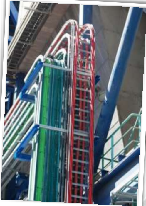
Litoral Power Plant (ENEL) Carboneras (Spagna)
