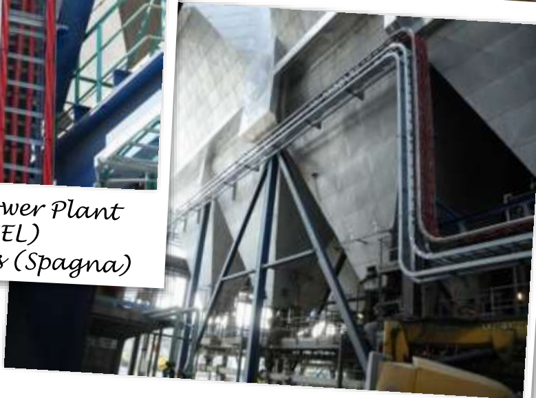
Litoral Power Plant (ENEL) Carboneras (Spagna)
