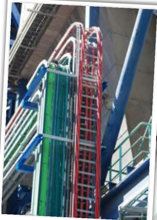
Litoral Power Plant (ENEL) Carboneras (Spagna)
