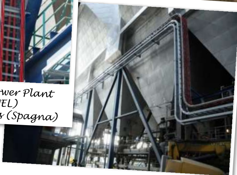
Litoral Power Plant (ENEL) Carboneras (Spagna)
